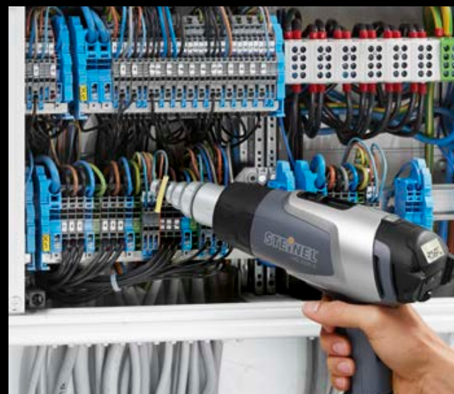
Shrinking cable sleeves in distribution cabinet
