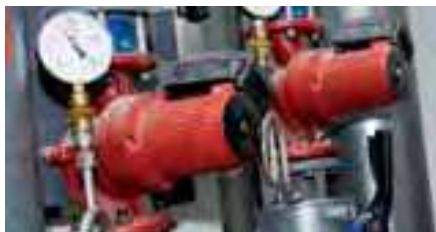
Actuators, valves, control cabinets
