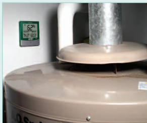
Monitoring Dew Point levels in a Basement for potential mold growth.
