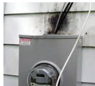
Service entrance destroyed by a surge
