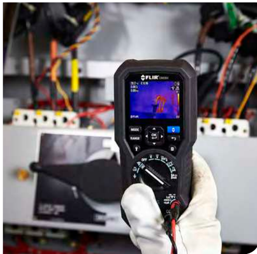
Thermal scan of an electrical panel
