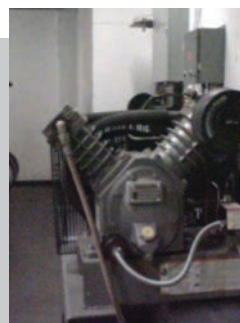
Air Compressor – Full Visible
