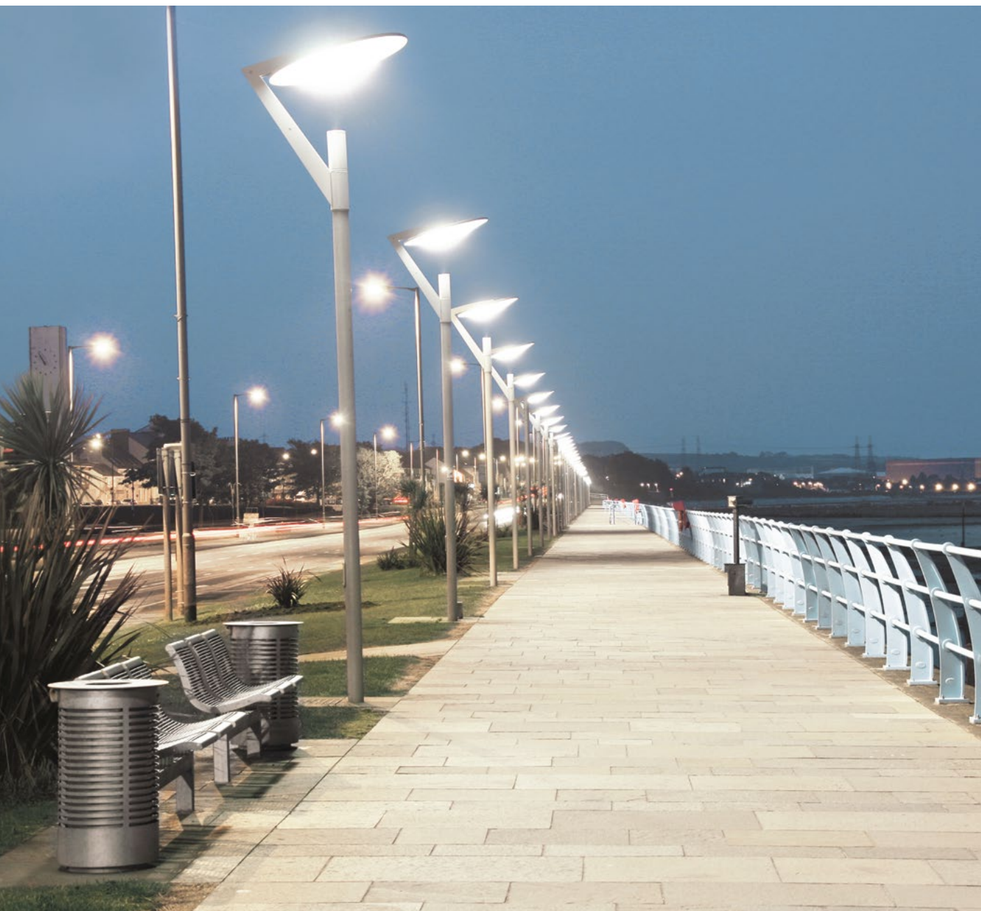
Modern street lighting with high reliability and long lifetime
