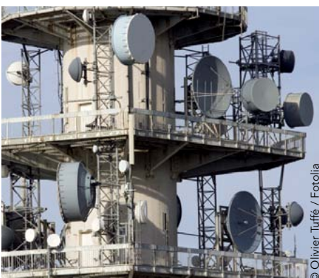
Telecom - Data infrastructure
