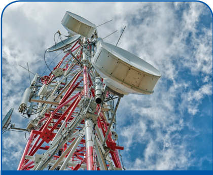
Telecom -Data Infrastructure
