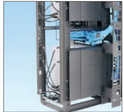
Panduit 4 post rack thermal ducts shown in a dual Nexus 7009 switch deployment.
