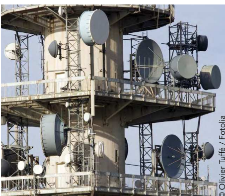
Telecom - Data infrastructure
