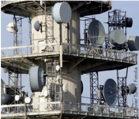
Telecom - Data infrastructure
