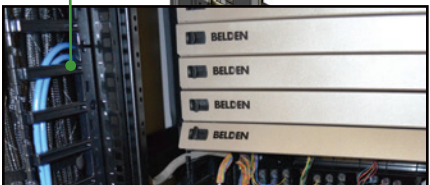
Vertical Manager shown in cabinet
