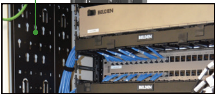
Lacing Panel shown in cabinet
